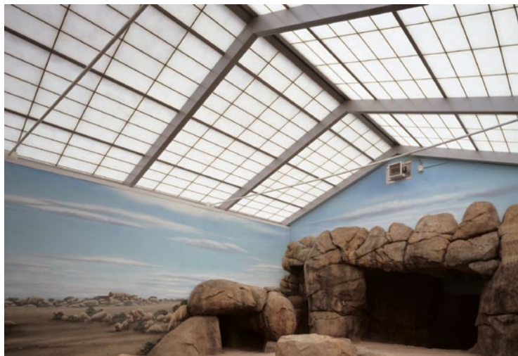
Nanogel-filled insulated glazing units at the Milwaukee Zoo.
